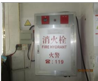
Photo of fire safety equipment Fire hydrant.JPG
