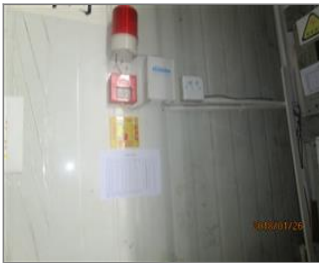
Photo of fire safety equipment Fire alarm.JPG
