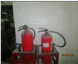
Photo of fire safety equipment Fire extinguishers.JPG
